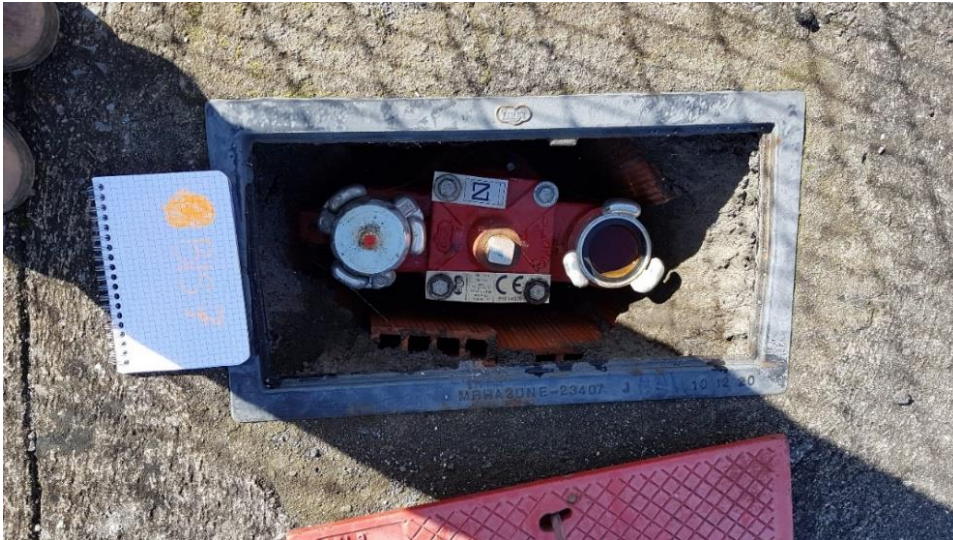
Illustration 4. Example of hose faucet without a meter
